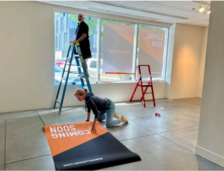
Andria Friesen and crew installing COMING SOON signage on behalf of Sun Valley Contemporary Gallery
